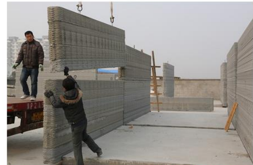
A house is constructed using a 3-D printing process. See more photos of the 3-D homes being constructed. WINSUN NEW MATERIALS
